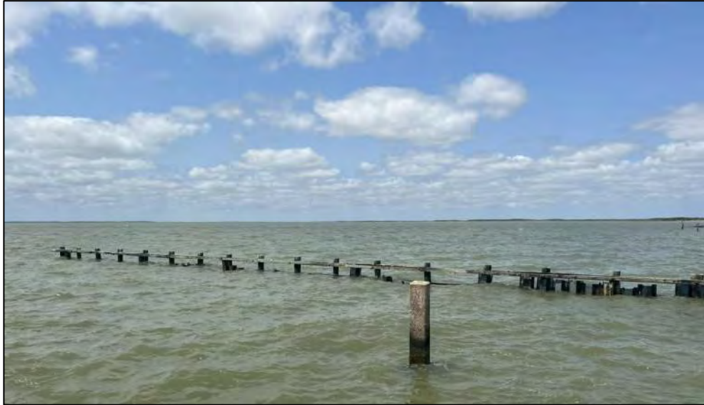
Figure 4 Failed vinyl sheet pile breakwater
