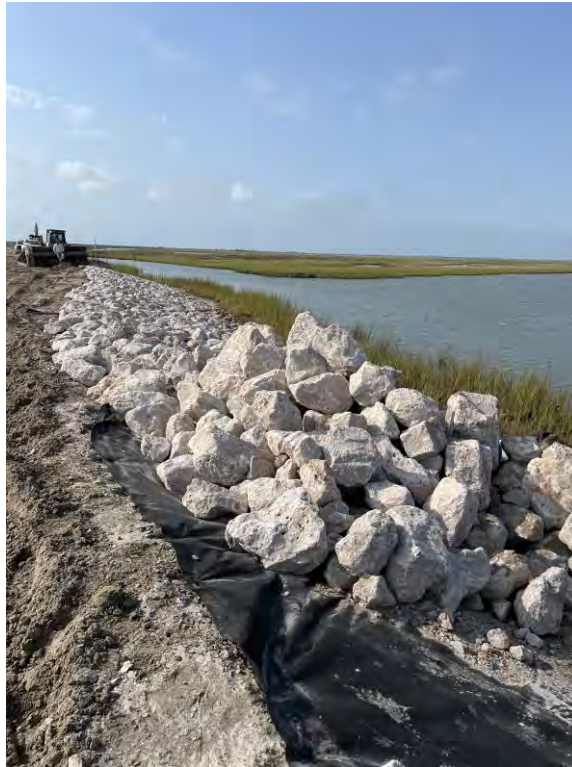
Photo 5. Placement of riprap and geotextile on west side up to approximately STA 4+00 (facing south).
