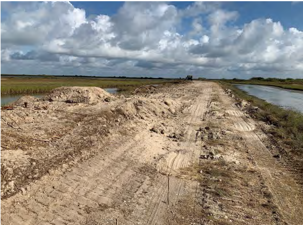
Photo 2. North end of cleared sand stockpile near B-SR-1 (looking north). Note area that has removed sand for placement in breach closure.
