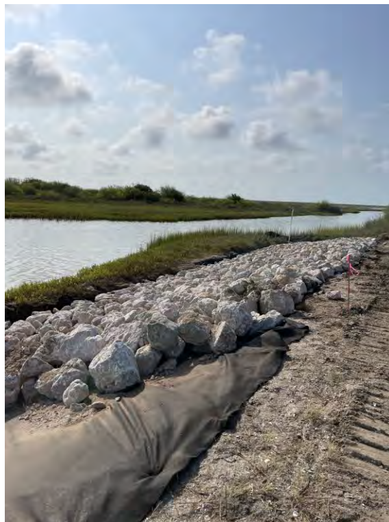
Photo 4. Placement of riprap and geotextile on east side up to approximately STA 3+50 (facing south).
