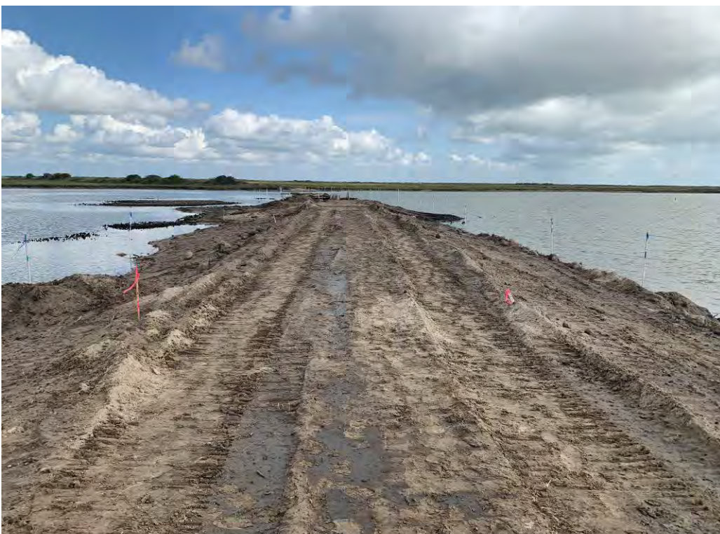
Photo 4. Placement of stockpile sand to fill levee breach on south end of breach (looking north) at approximately STA 100+00.
