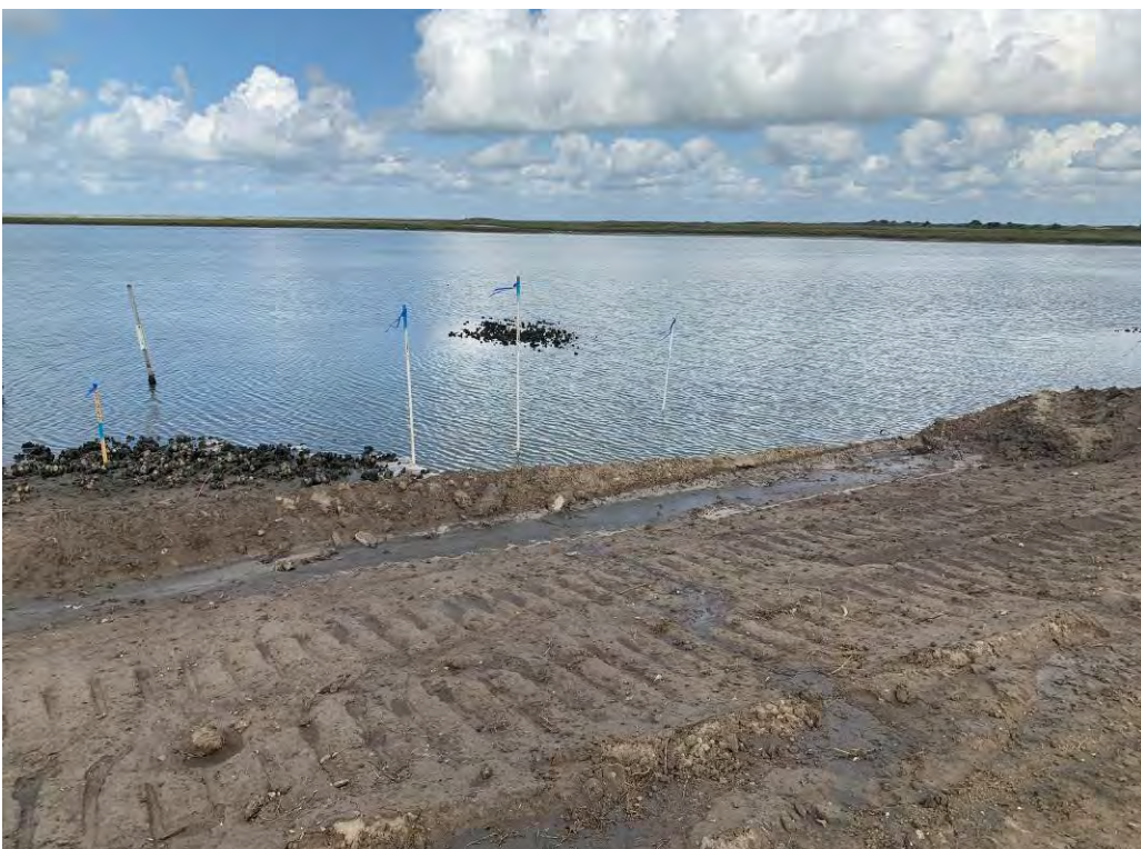
Photo 6. Tall poles mark initial culvert location at approximately STA 2+00 (looking west). Culverts to be shifted 5-10 feet north to avoid impacts to oyster resource.
