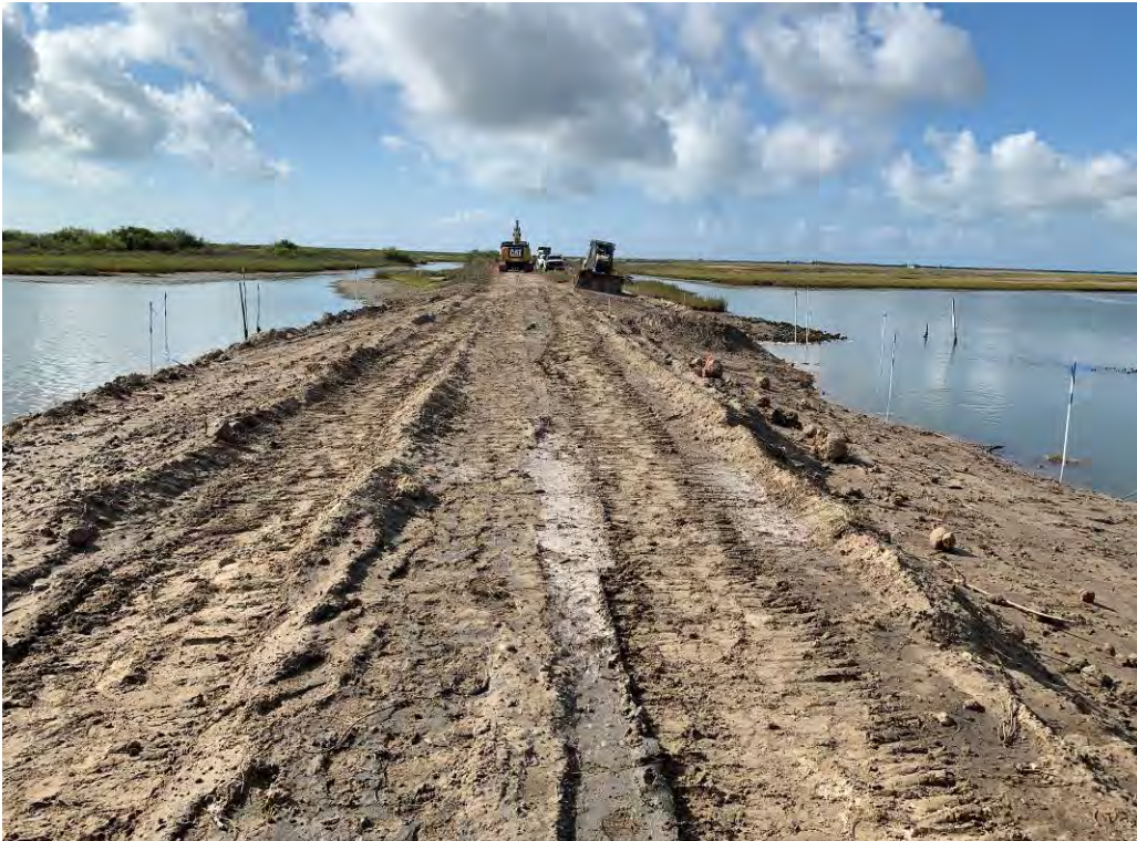
Photo 3. Placement of stockpile sand to fill levee breach on south end of breach (looking south) at approximately STA 150+00.
