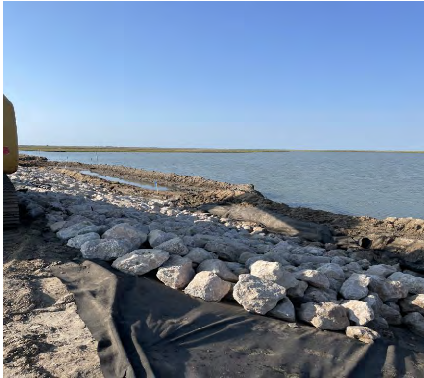
Photo 3. North extent of stone and geotextile placement (STA 4+50) on west side of B-SR-1 (facing south).
