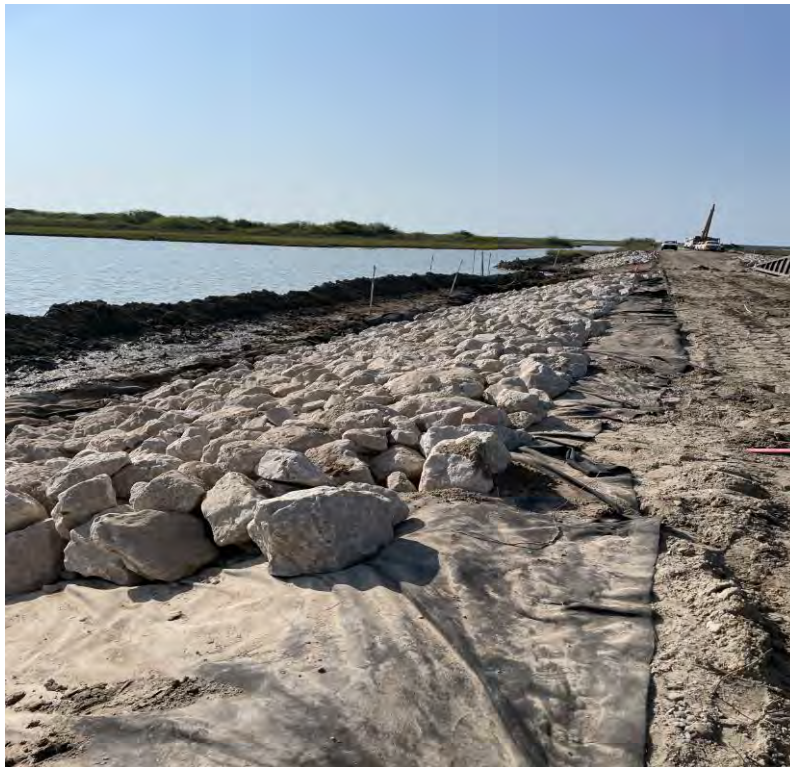
Photo 2. North extent of stone and geotextile placement (STA 4+00) on east side of B-SR-1 (facing south).
